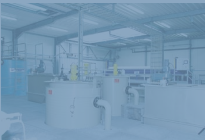
The new water effluent treatment plant at Holliday Pigments' main manufacturing site in Comines, Northern France.
